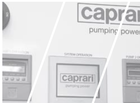
Pump Control Technology
