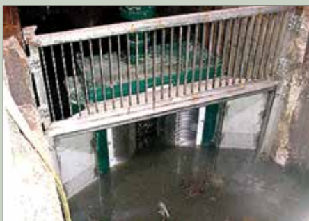
Overflow Bar Screens
